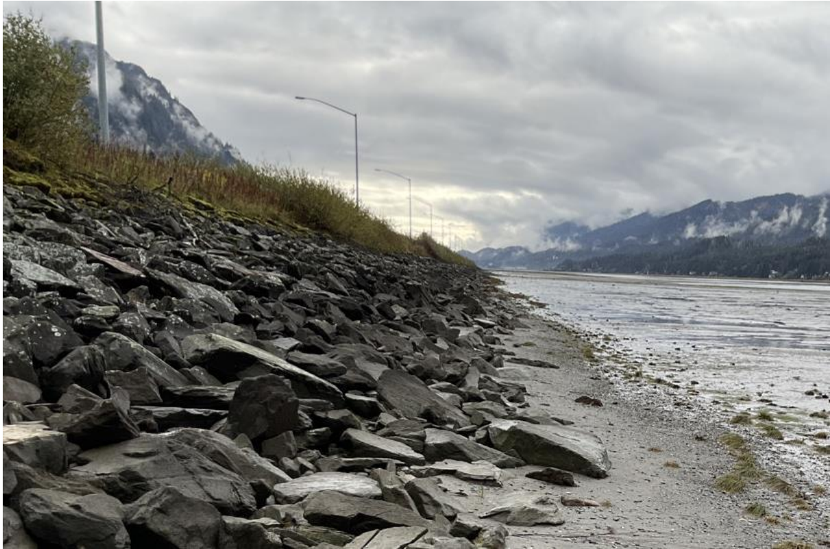
Riprap bank armoring along Gastineau Channel in Survey Area A9, facing south.
